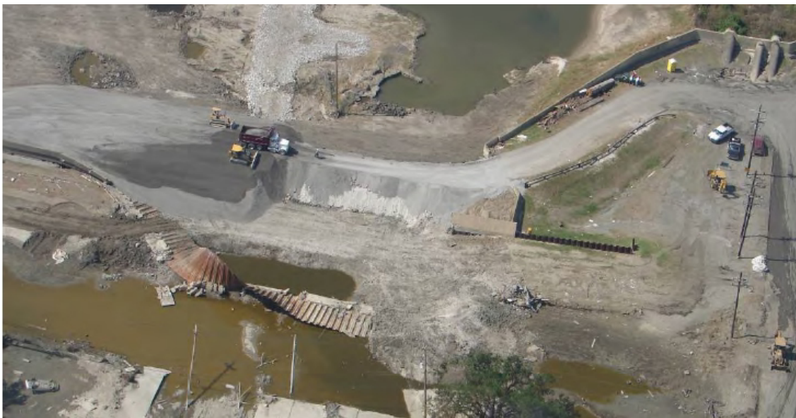
Figure 14. Aerial view of the north breach on Industrial Canal. Photo by L. Harder - Independent Levee Investigation Team Draft Final Report (2006).
