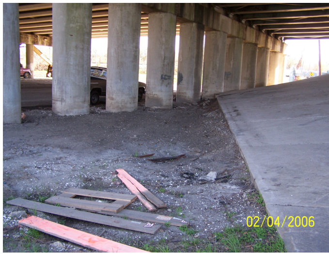
Figure 41. Erosion around the support structures for I-610 near Orleans Canal on Marconi Ave.
