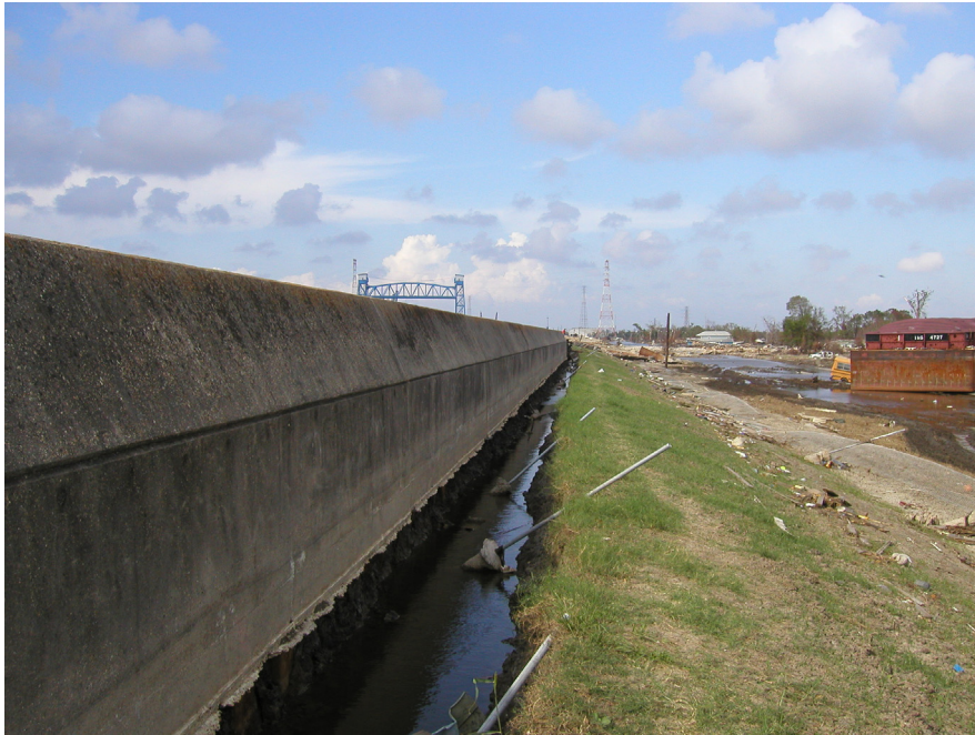
Figure 11. Looking North along the floodwall of the Industrial Canal levee showing trenches eroded by water from the Industrial Canal that overtopped the floodwall. Photo from U.S. Army Corps of Engineers IPET web site, taken October 4, 2005.
