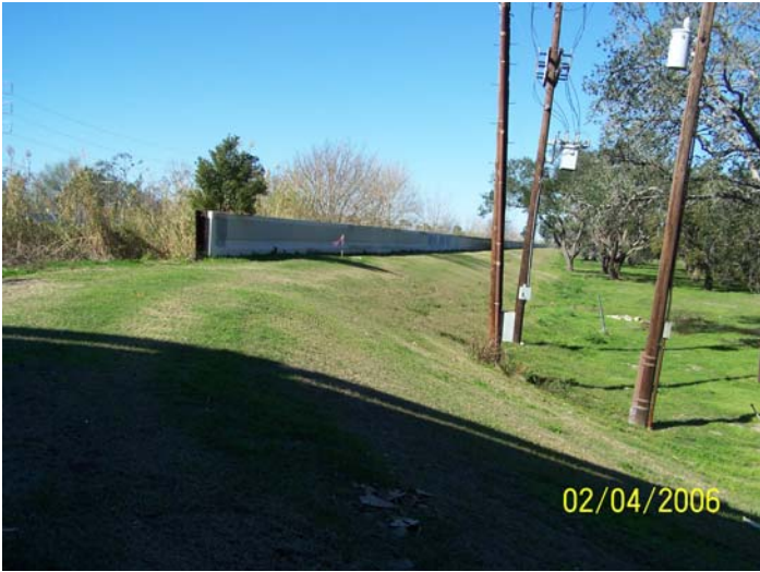
Figure 53. End of floodwall on Orleans Canal just north of I-610 overpass near Marconi Ave. (Stop 9)
