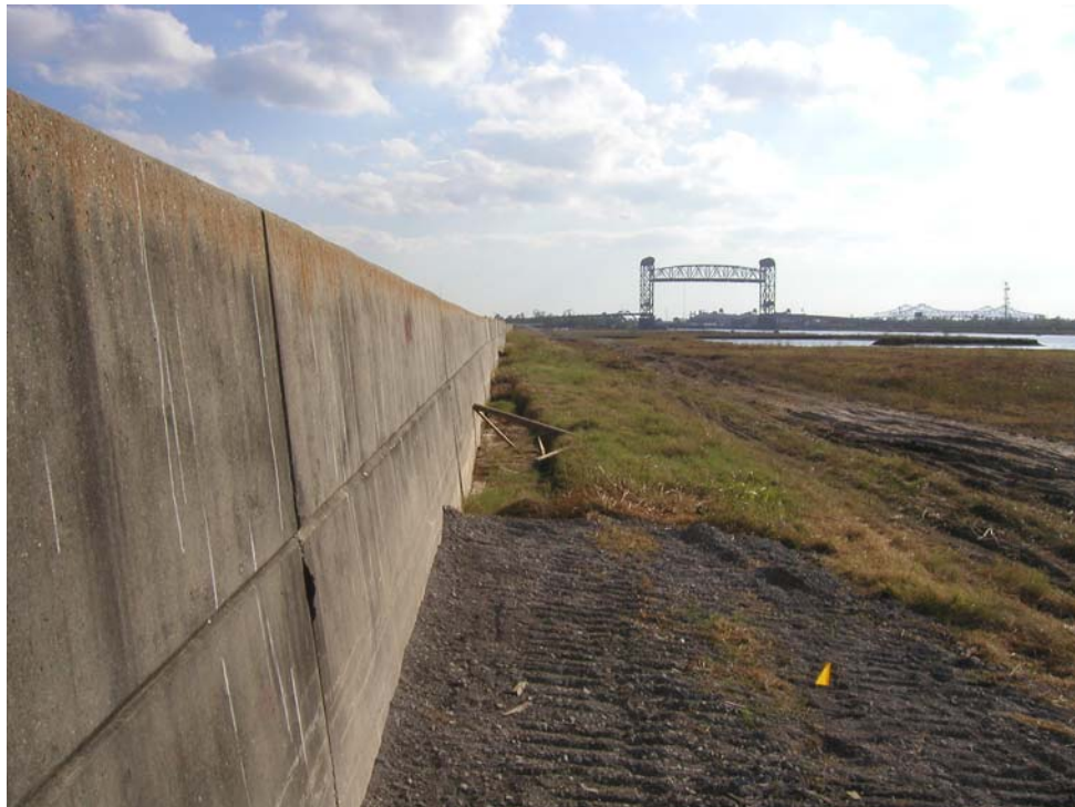
Figure 18. Looking South along the floodwall of the Industrial Canal on the inside of the floodwall between the two breaches showing the floodwall leaning toward the left (east) with a block of the levee next to the floodwall dropped down (near center of picture). Claiborne Ave. Bridge in right center. Photo from U.S. Army Corps of Engineers IPET web site, taken October 4, 2005.
