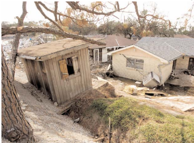
Figure 37. Child's clubhouse behind the Cantrell home on Pratt Drive uplifted along the west side of the London Avenue Canal near the breach (Stop 5). Note the fractures beneath and in front of (right side in photo) the clubhouse. Gray material at base of tree is gravel used in the repair of the breach. Source: Times-Picayune Tuesday, October 4, 2005. See reference to article by John McQuaid, same date
