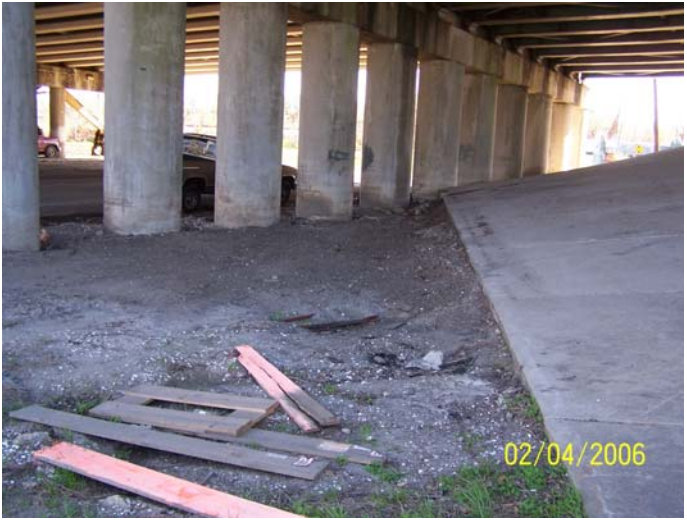
Figure 54. Erosion around the support structures for I-610 near Orleans Canal on Marconi Ave (Stop 9).
