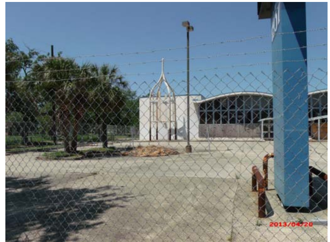
Figure 26. Church at the corner of St. Anthony and Mirabeau showing the standing water line and rusted church steeple.
