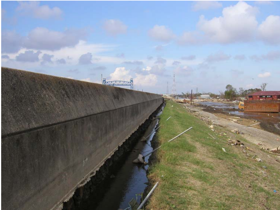
Figure 17. Looking North along the floodwall of the Industrial Canal levee showing trenches eroded by water from the Industrial Canal that overtopped the floodwall. Breached section is just beyond the barge and barely discernable in this view. Florida Avenue Bridge (blue) in upper center. Photo from U.S. Army Corps of Engineers IPET web site, taken October 4, 2005.
