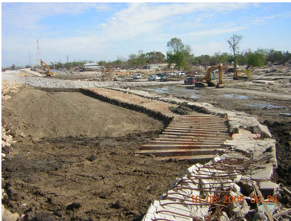
Figure 15. Floodwall and sheet piling strewn into Lower 9 th Ward at the southern (larger) breach on the Industrial Canal. Photo from U.S. Army Corps of Engineers IPET web site.
