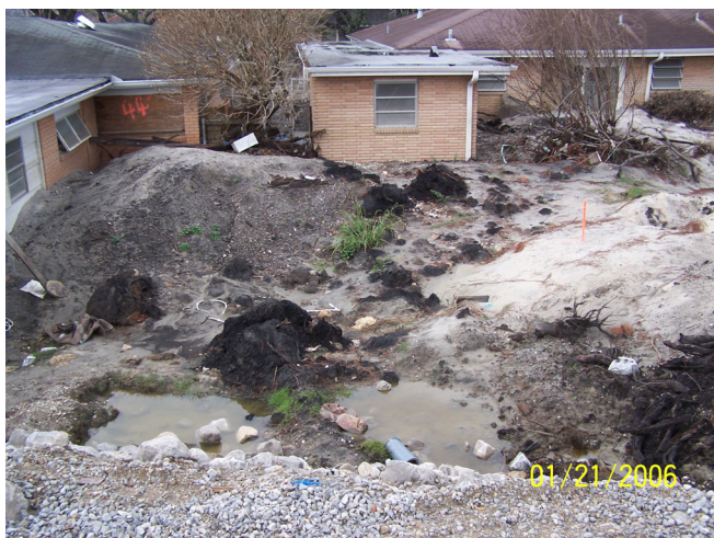
Figure 36. Sand deposits and peat blocks (black) behind homes on Pratt Drive at the North breach of the London Ave. Canal. Note the sand boil on the right. Gray material in the foreground is gravel used in the repair of the breach.
