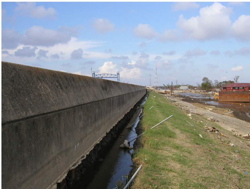
Figure 11. Looking North along the floodwall of the Industrial Canal levee showing trenches eroded by water from the Industrial Canal that overtopped the floodwall. Photo from U.S. Army Corps of Engineers IPET web site, taken October 4, 2005.
